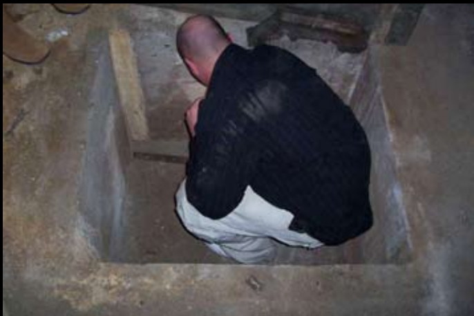
Jason investigating the large square cement hole in the basement.
